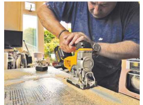
▲ A jigsaw often earns its keep in kitchen fitting such as cutting out for sinks and hobs
